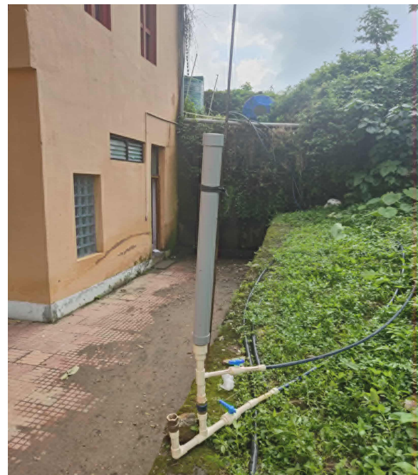
Fig. 3: Ram pump set-up site, showing the supply tank, the drive pipe alignment and the elevation difference between the water source and the pump
